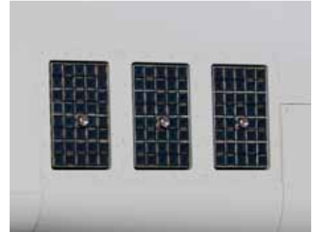
BOP Dispensers installed
